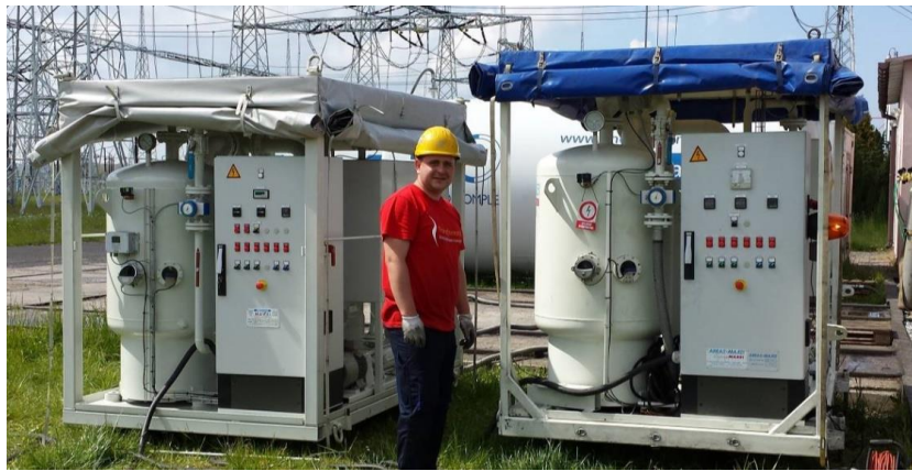
Fig. 5. MAS-600 oil processing system warming up oil that circulated through the transformer.
