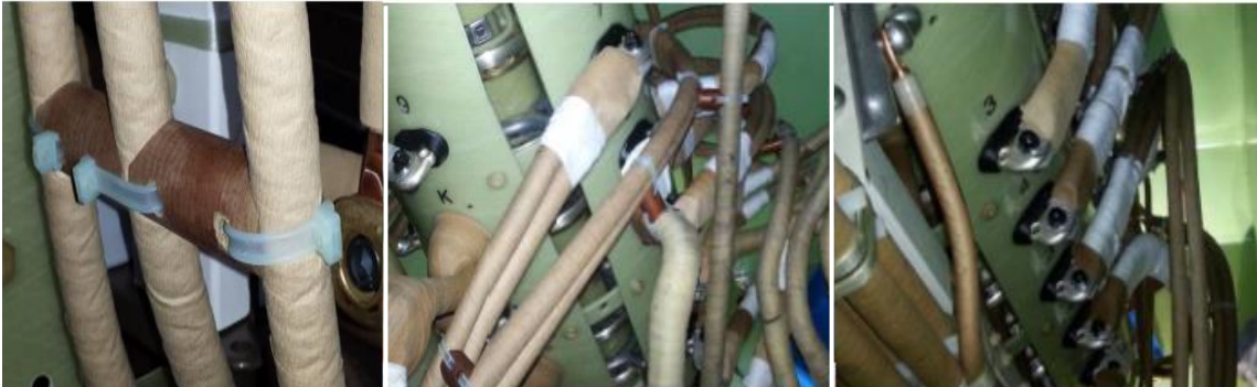
Fig. 2 Leads connecting OLTC selector to the tap-winding. Joints between original lead and its extension were clamped and insulated with wrapped tape, inside the tank. Spacers ensured the distance between the leads calculated according to their respective voltage-difference.
