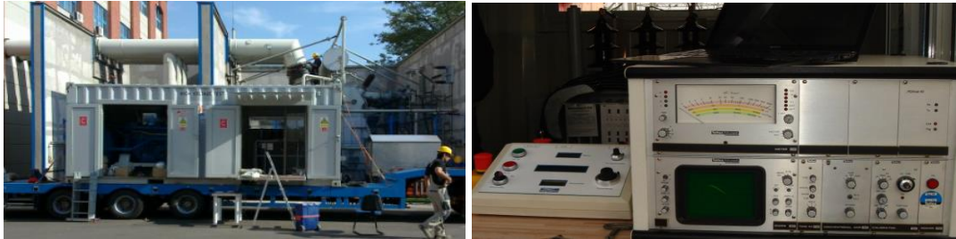
Fig.1. Mobile motor-generator set on a trailer and Partial Discharge level measured by Tettex 9120.
